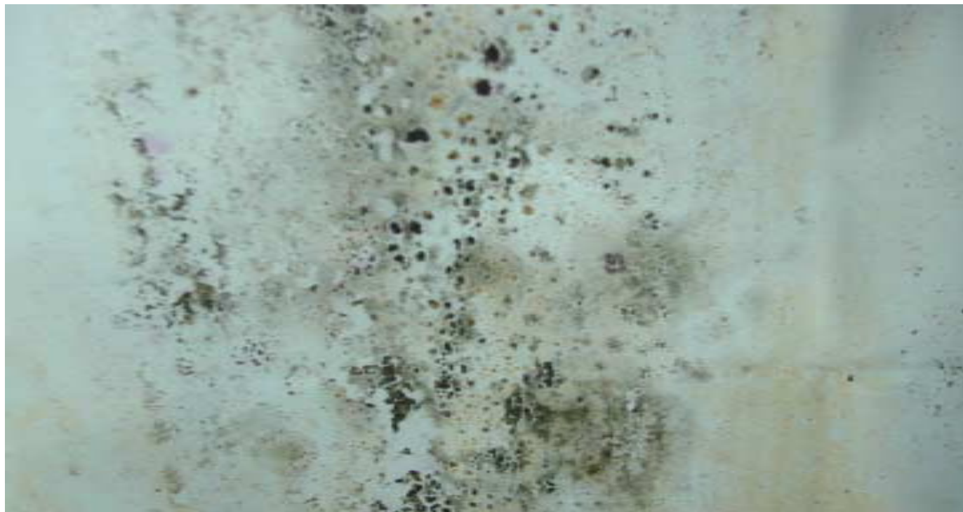
(Mold on the bath curtain)
